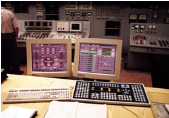
Safety parameter display systems provide critical information on plant conditions to control room personnel during emergencies. (Photo courtesy of Energoatom.)
