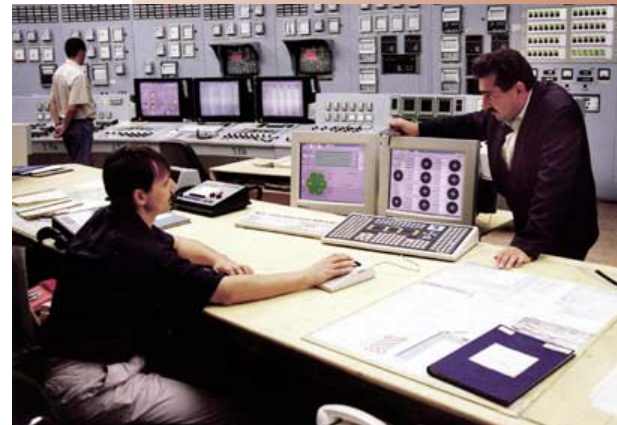
Heorhiy Balakan, shift supervisor (standing), and Stepan Stoykov, senior reactor operator. Plant operating staff check values of critical safety parameters at South Ukraine Unit 1. Values are displayed on two safety parameter display system computer monitors in the reactor's main control room.
