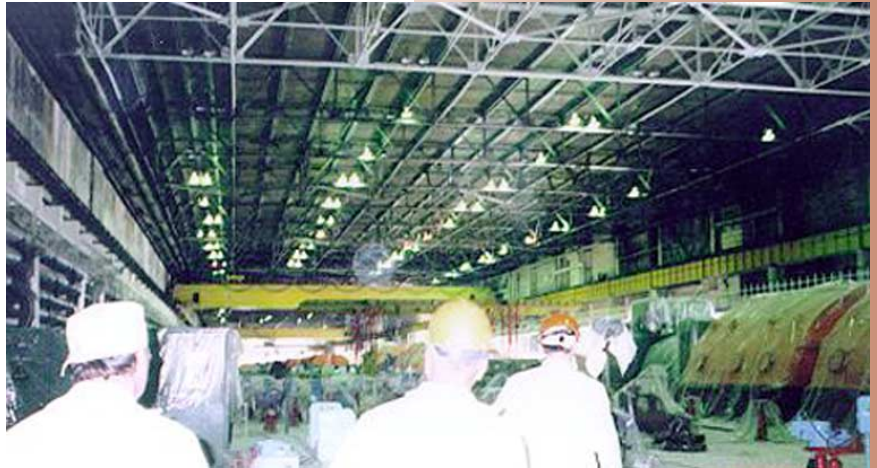
During the spring of 1998, workers applied a fire-resistant coating to the structural steel in the Chornobyl Unit 3 turbine building. As shown in this photo, all of the equipment and the floor of the building were covered with plastic while the material was applied. The coating (which is white and can be seen in this photo) is to prevent damage from a fire that could result in failure of the roof—as was the case in the 1991 fire in the Chornobyl Unit 2 turbine building.
