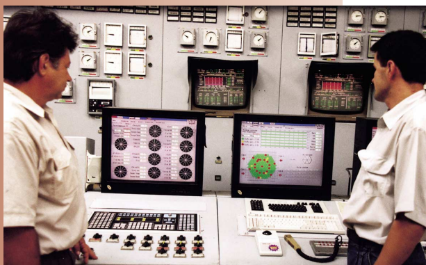
Aleksandr Priamikov, senior reactor operator (left), and Valeriy Gonchar, reactor operator, check safety parameters on a display system at South Ukraine Unit 1. The system began operating in June 1998.
