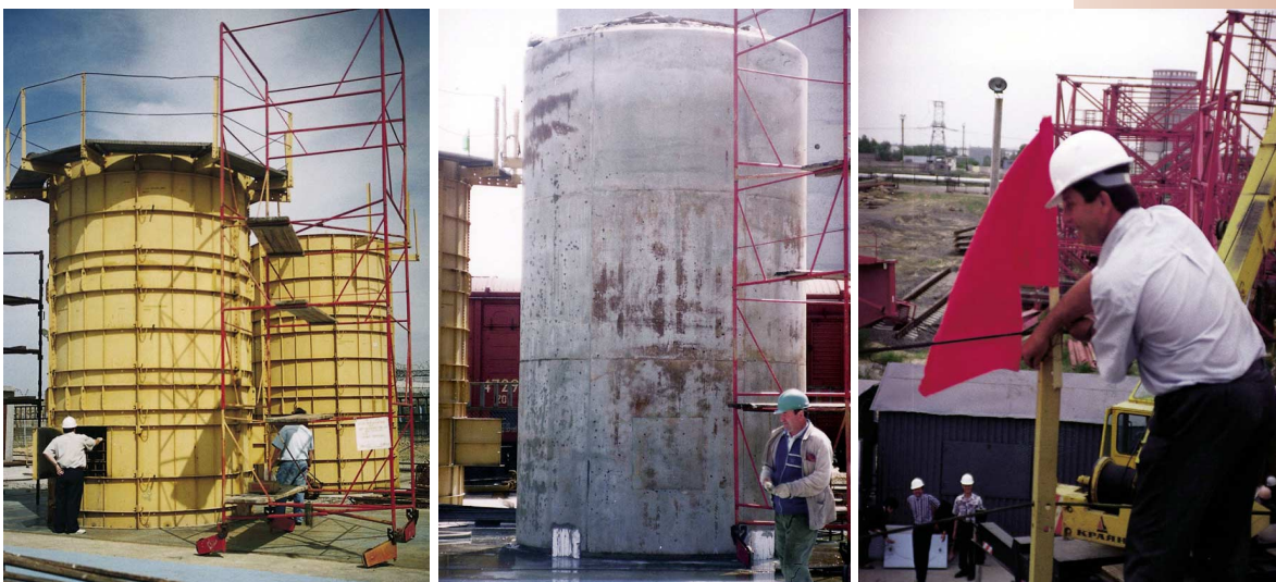
The spent-fuel dry-cask storage project is enlarging the storage capacity at the Zaporizhzhya nuclear power plant. Workers are shown erecting the ventilated concrete cask (left), near a cask after removal of concrete forms (middle), and attaching the approval flag after acceptance of the first cask in May 1998 (right).
