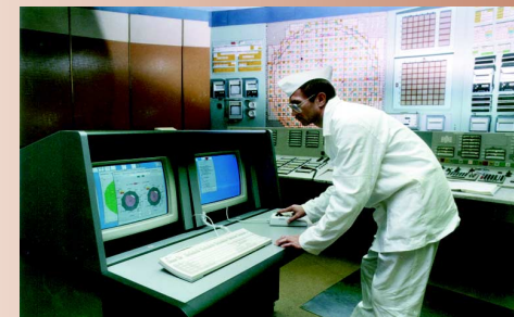
Safety parameter display systems, like the one at the Kursk nuclear power plant, provide key information for preventing accidents.
