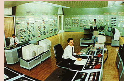
Reactor operators train on full-scope control room simulators, like this one at the Balakovo nuclear power plant.
