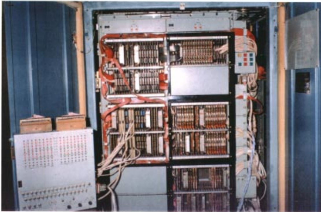
Frame-mounted «YBK» (Controlling computing complex) of System «Э4 АСУТ-1000P(2P)» (Electronic part of automated systems for controlling technological processes), systems of automatic regulation and functional-group control
